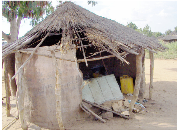
Figure 1 Elderly widow's dilapidated house before
